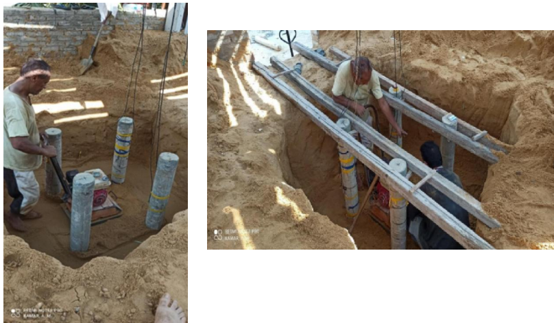
Fig (17) Placing piles and keeping the distance between piles (5-diameters from center to center) – group of four piles
