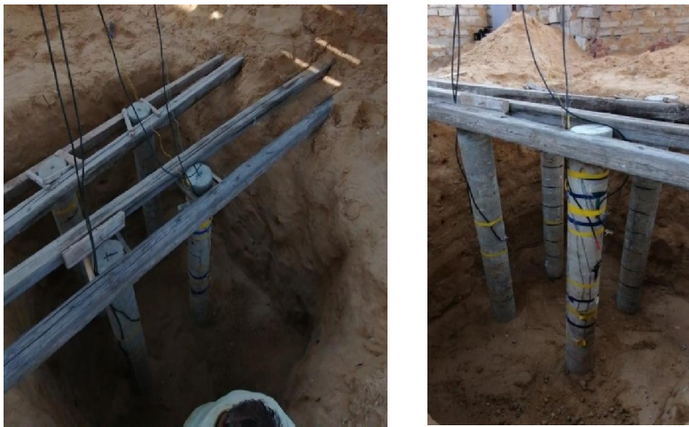
Fig (13) Placing piles and keeping the distance between piles (4-diameters from center to center) – group of four piles
