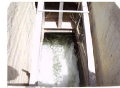
Figure 13: 370 CUSEC Water from Hub Dam to Main Canal Proposed Site for MHPP-1
